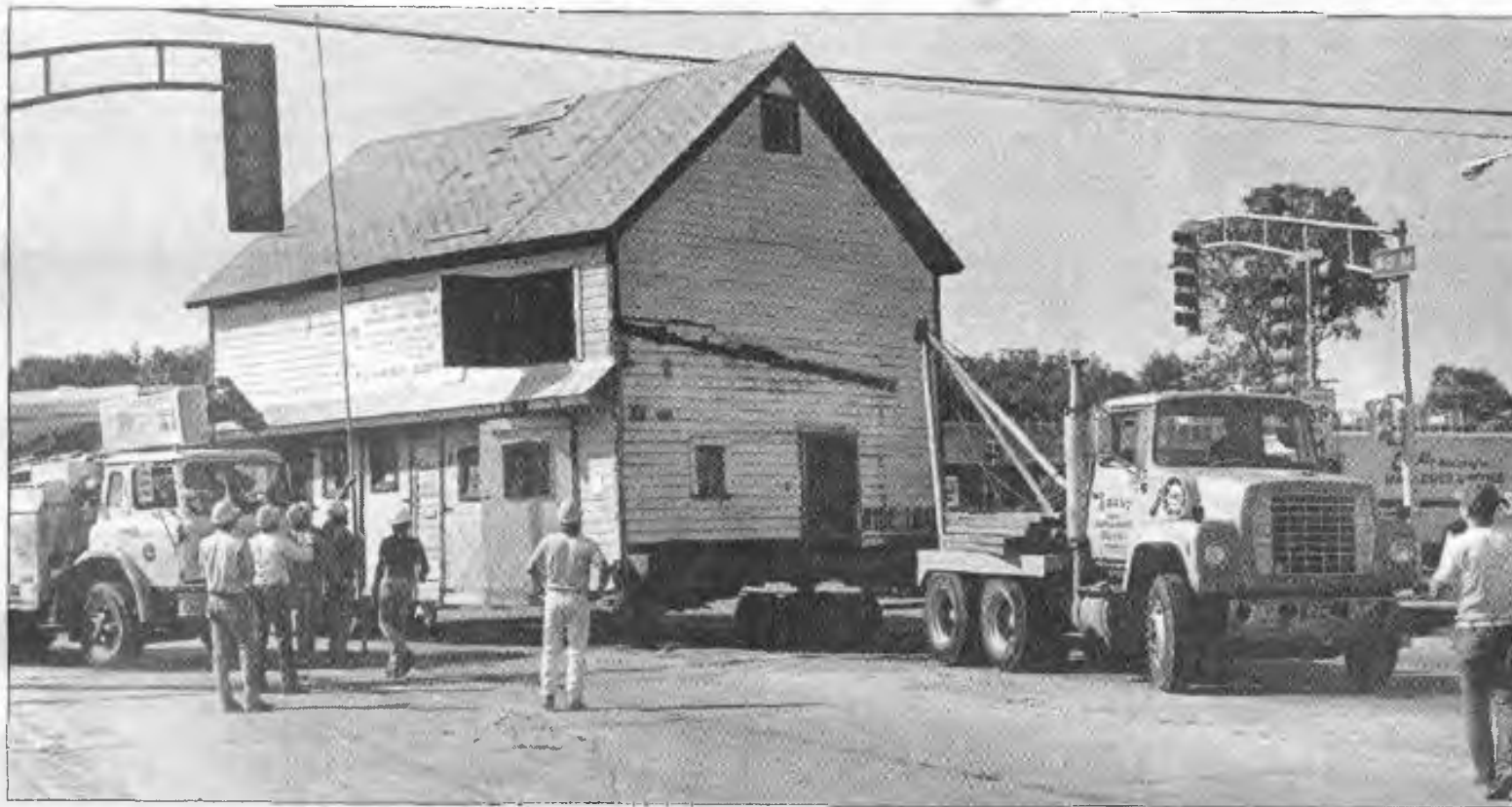
The toughest part of the crosstown journey for the former barn is this tricky turn from Dundee Road onto Wolf Road.
